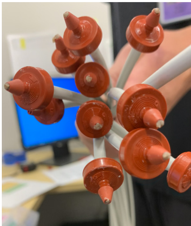
Figure 24. Clogged drip irrigation emitters.
