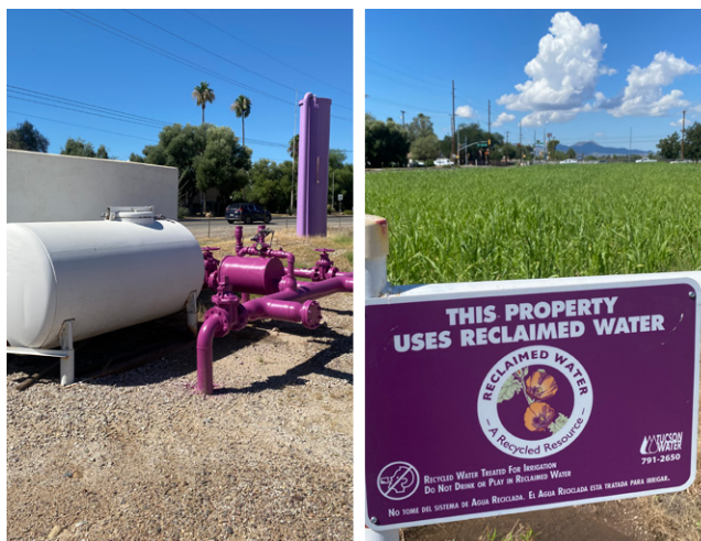
Figure 45. Purple pipes indicating recycled water at the Controlled Environment Agriculture Center, University of Arizona.
