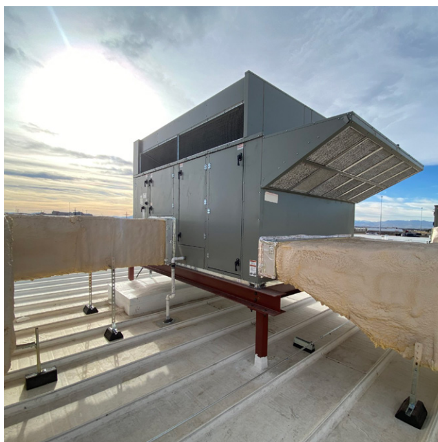
Figure 18. Rooftop HVAC/Dehumidification unit with insulated ductwork and condensate drain.
