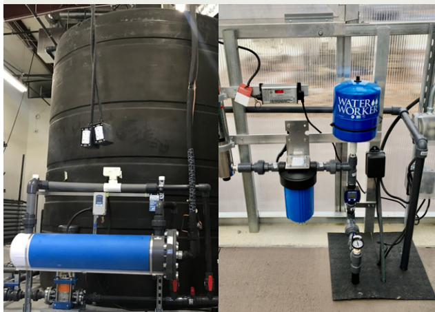
Figure 36. Water tank with UV light disinfection loop (left) and UV loop on underground rainwater tank.
